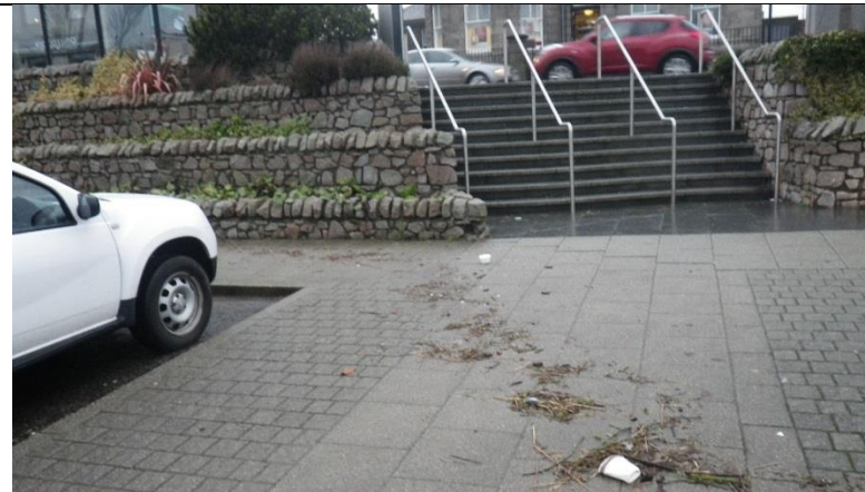
Photo 03: Market Street Car Park, with debris line evident at base of steps to Market Street (taken 08/01/16)
